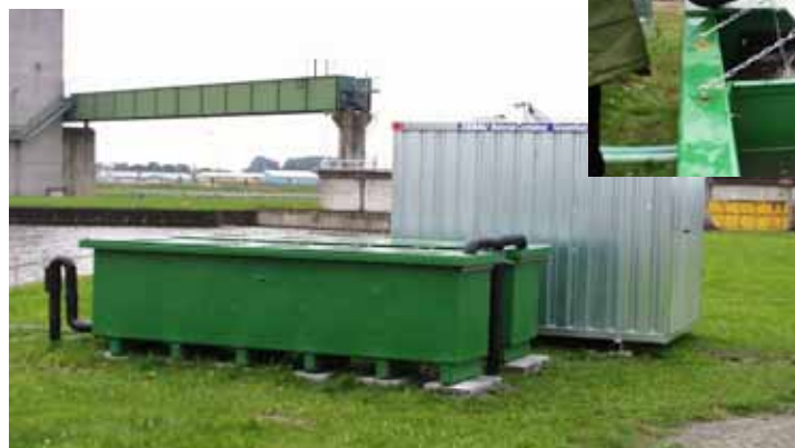
LEFT: MIGROMAT SYSTEM AT HYDROPOWER STATION ALPHEN. SOURCE: KEMA, 2002.
